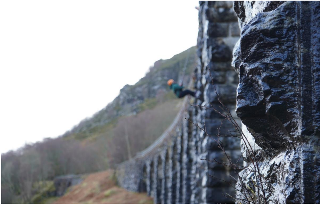
Image Description: A participant is abseiling down the face of a viaduct.
